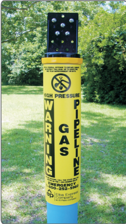
H41 Cathodic Test Station with HDPE Sleeve
