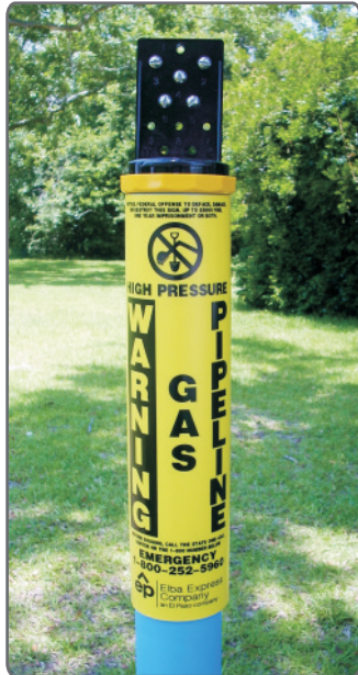
H41 Cathodic Test Station with HDPE Sleeve
